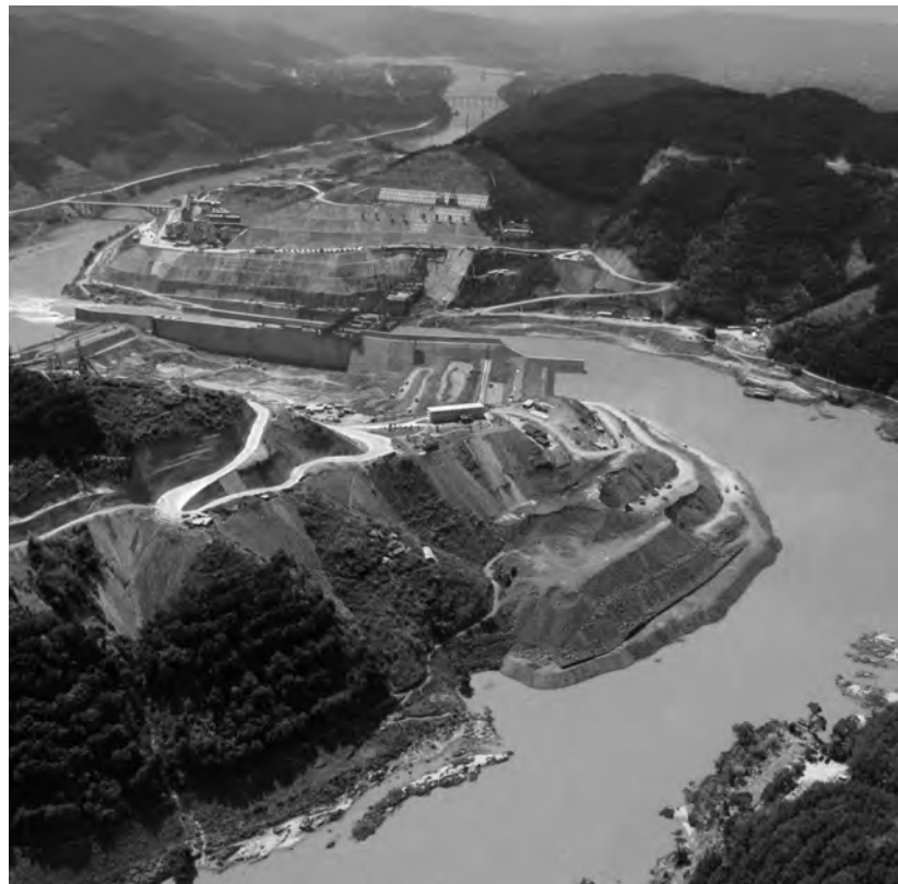
Construction of the Jinzhong hydropower plant on Lancang River (part of the Mekong River in Yunnan Province, China). © 2005 Imaginechina.
