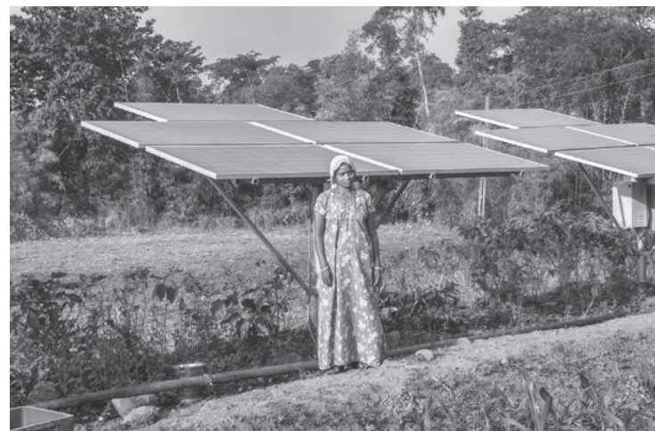
Villager standing in front of solar irrigation panels in Dabka Village. Source: Photo by Trupti Mehta.
