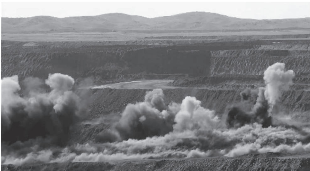
The Ukhaa Khudag (UHG) coal mine, located in Mongolia's south Gobi Desert, is one of the largest open-pit coal mines in the world. UHG is owned and operated by the private Mongolian Mining Corporation (MMC). The majority of coal is used for steel production. Source: Screen capture from the documentary Mongolia's Mining Boom (2012) at https://tinyurl.com/p523eunc . © Journeyman Pictures.
