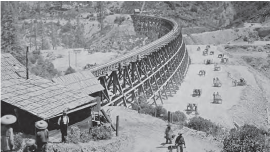
Chinese workers on the construction of a hugh trestle for the transcontinental railroad. Source: Screen capture from the short documentary, The Work of Giants . Source: YouTube at https://tinyurl.com/3a5yp2wb .
